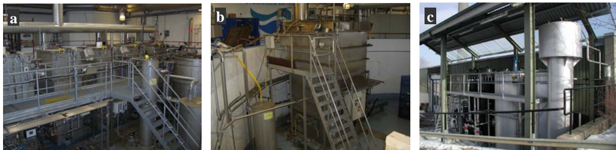
Figure 1. Pilot plant lines at Hammarby Sjöstadverket; a) traditional activated sludge process with sedimentation, b) membrane bioreactor (MBR) and c) UASB-reactors and sludge digesters.
